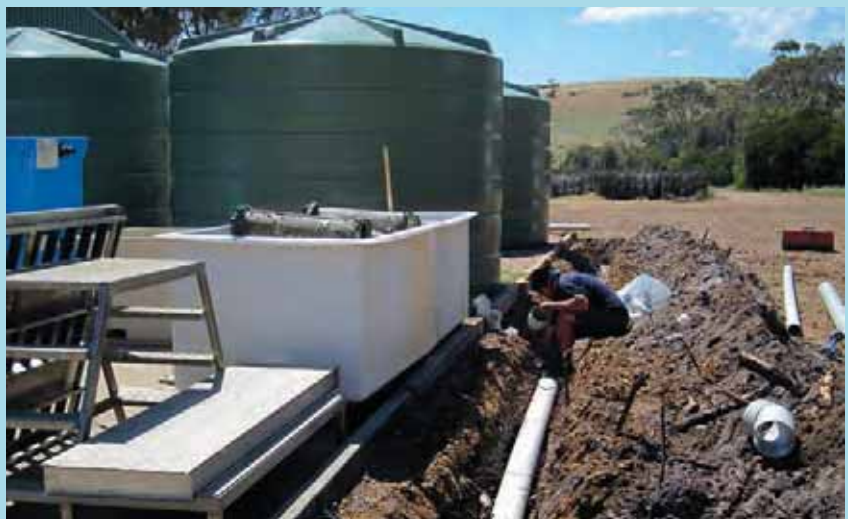
Top: Rack building progress on new farm; Above: Installation of new water tanks at new farm facility
